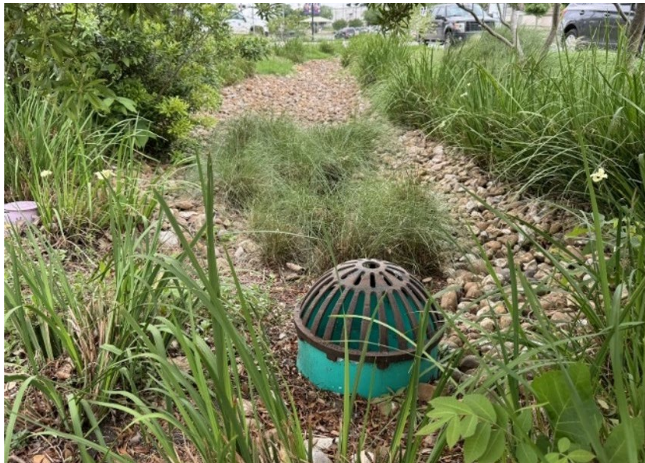
Figure 11-4. Stormwater overflow structure with domed debris grate
